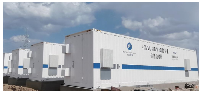
Inner Mongolia | wind power distribution and storage | 80MWh
