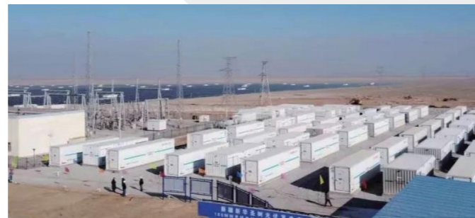
Xinjiang | Wind and solar energy distribution and storage | 315MWh
