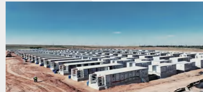
Ningxia | Shared Power Station | 400MWh
