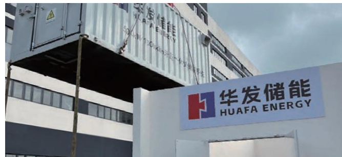
Guangdong | Industrial and Commercial Energy Storage | 4MWh
