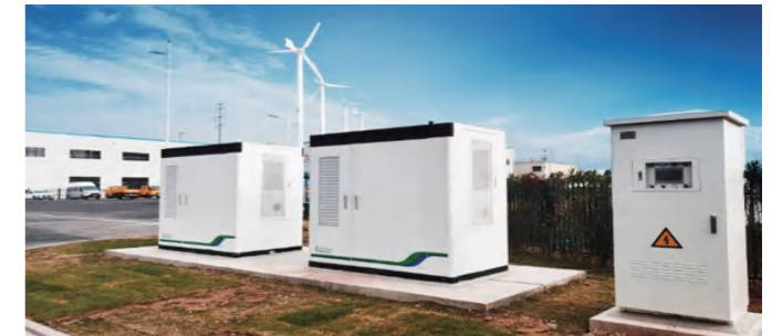
Anhui | Wind and solar power generation, energy storage, charging - supercapacitors - zero carbon park frequency regulation | 20KW/30S
