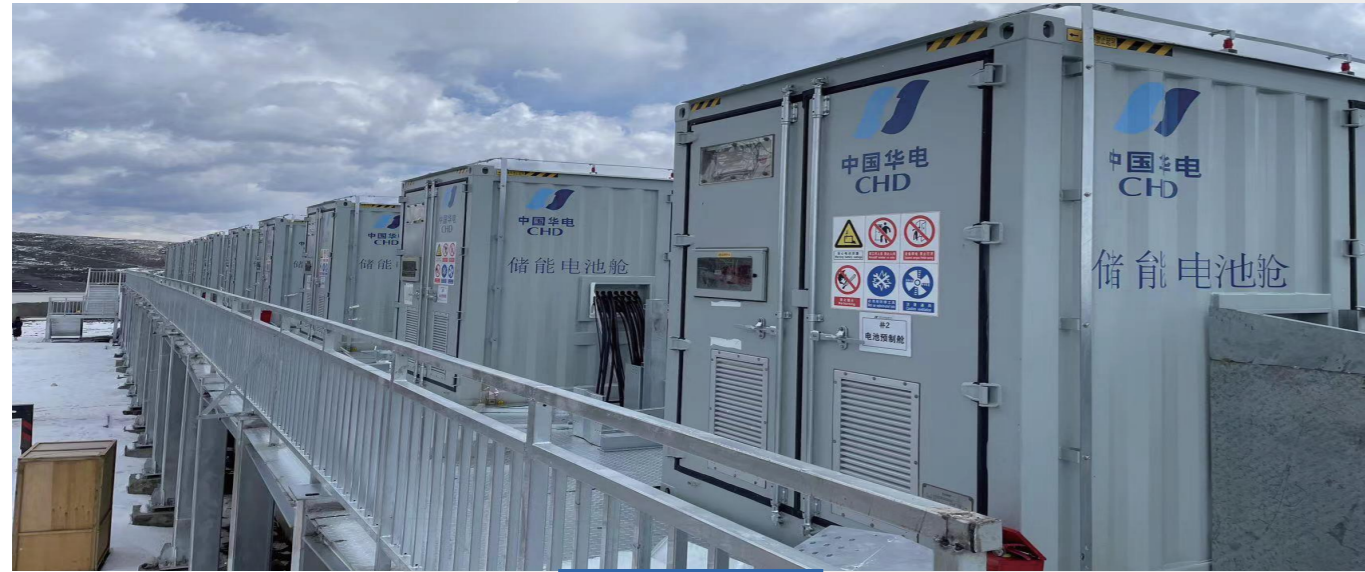
Sichuan | Photovoltaic Distribution and Storage | 50MWh
