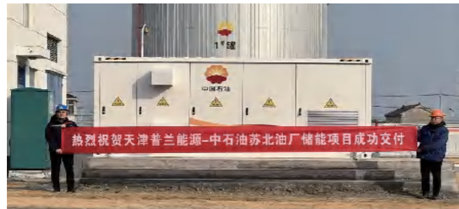
Jiangsu | Industrial and Commercial Energy Storage | 1.025MWh
