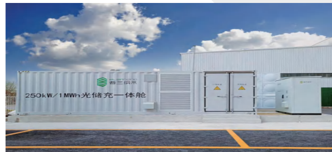
Tianjin | Optical Storage and Charging Microgrid | 1MWh
