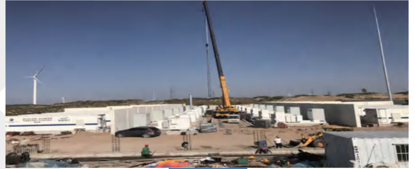
Inner Mongolia | Wind Power Distribution and Storage | 43MWh
