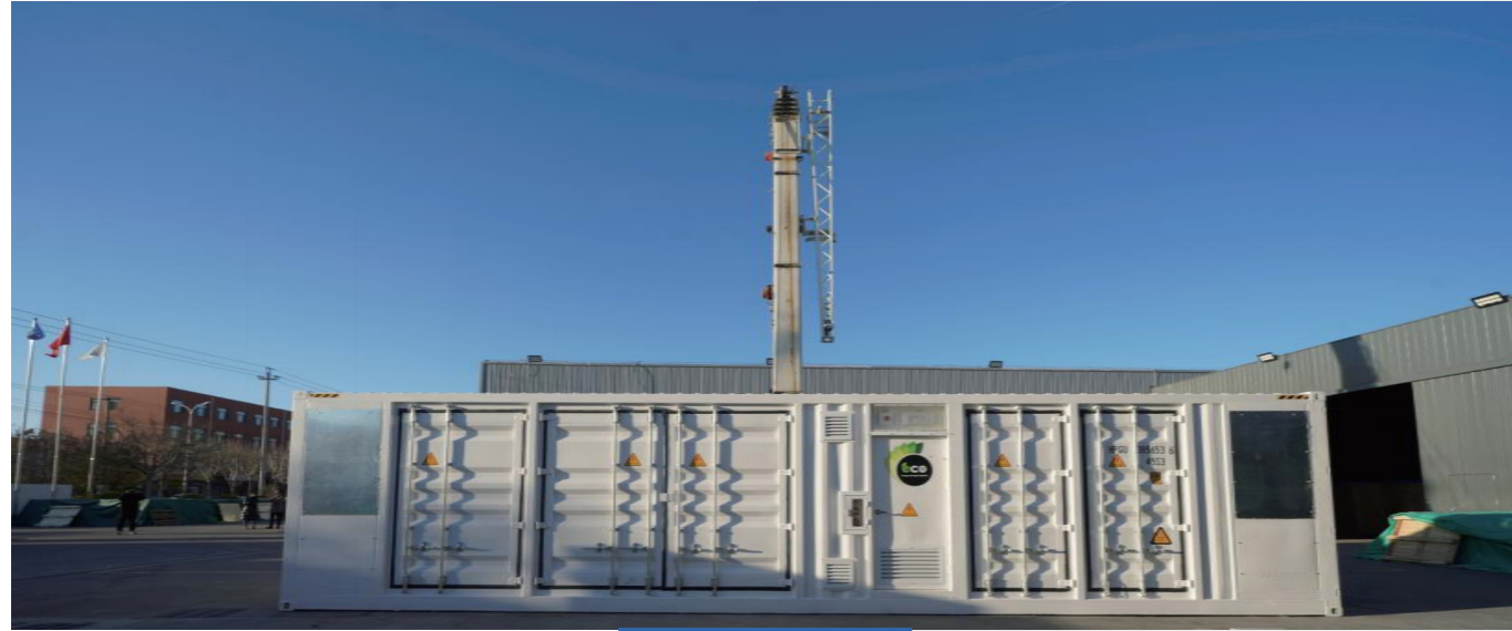
South Asia | Industrial and Commercial Energy Storage | 2.06MWh
