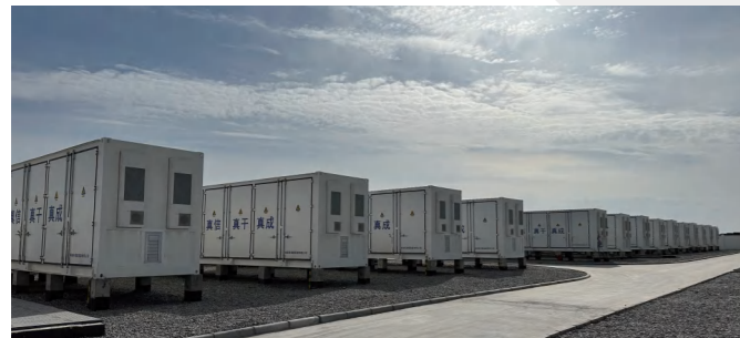
Xinjiang | Wind and solar energy distribution and storage | 200MWh
